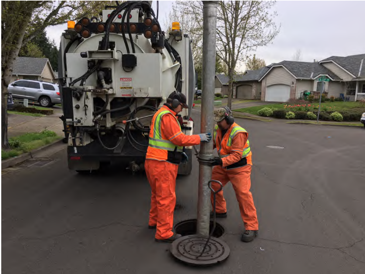
Cleaning Storm System
